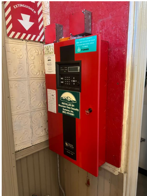
82 CRAFTSBURY ROAD – FIRE ALARM – FIRST FLOOR
