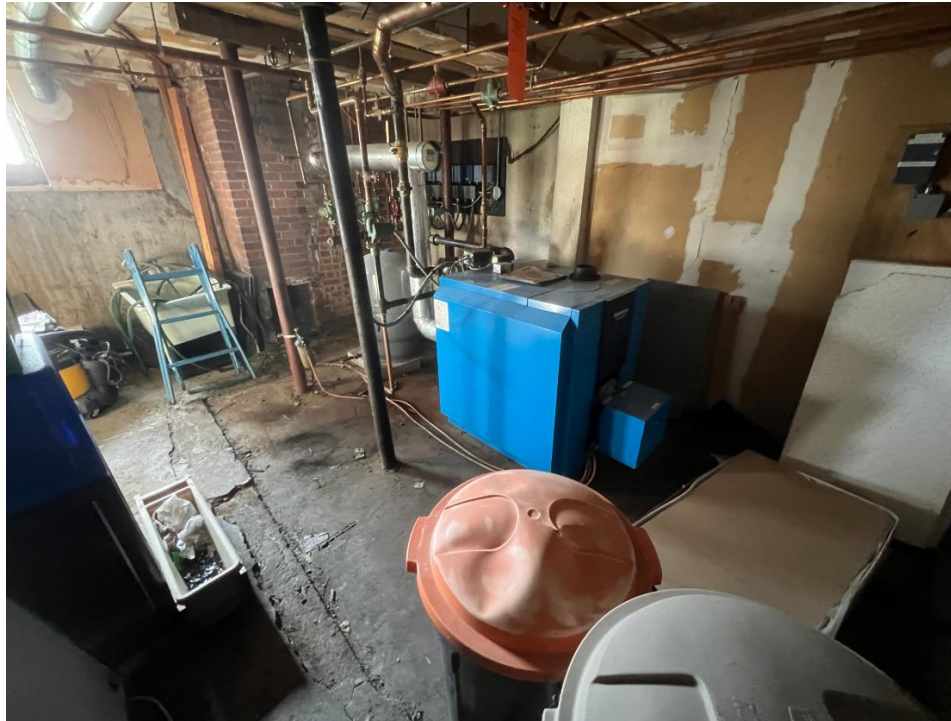
82 CRAFTSBURY ROAD – BASEMENT UTILITY ROOM
