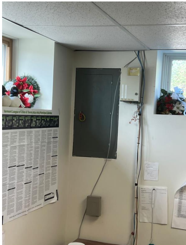
82 CRAFTSBURY ROAD – BASEMENT ELECTRICAL PANEL
