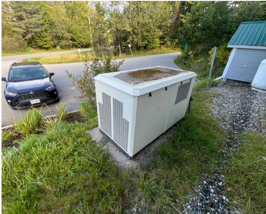
82 CRAFTSBURY ROAD - GENERATOR
