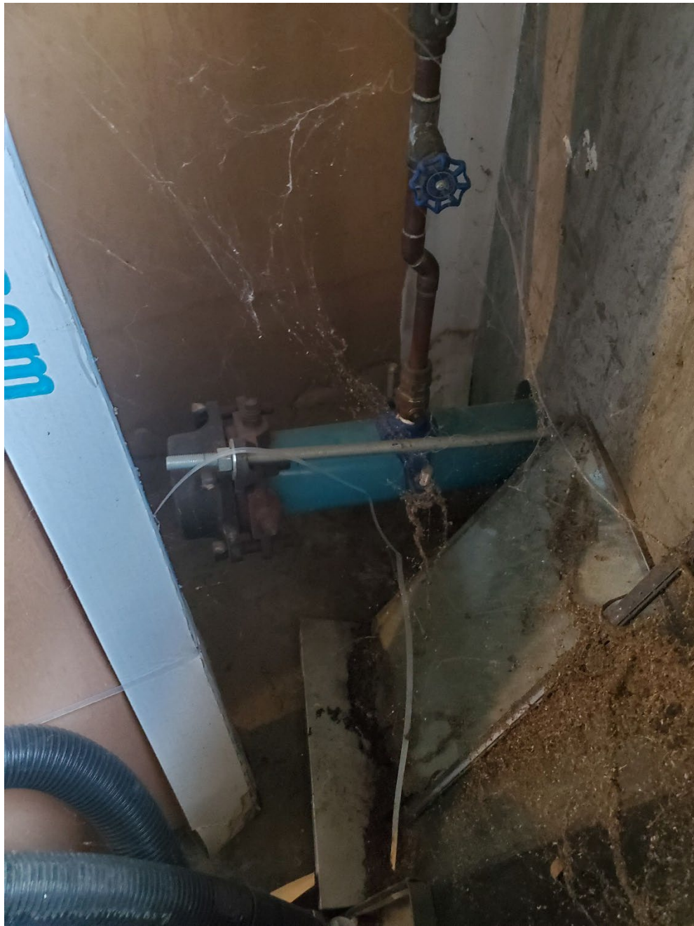
Photo # 1 Water service connection (4") into Town Hall building.
