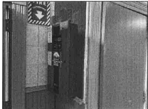
Interior, 1 st Floor – fire system
