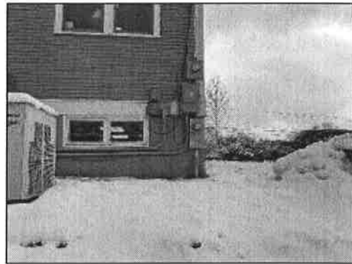
Exterior – electrical service and communications
