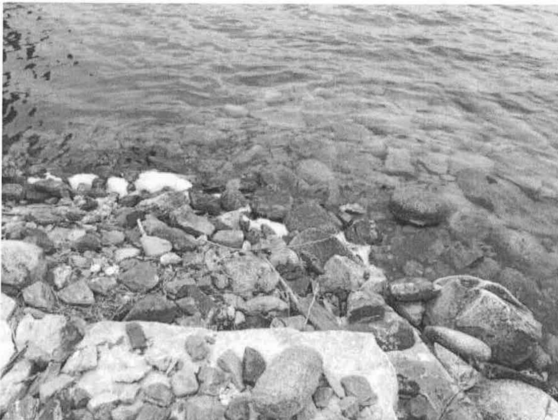
Left front corner, showing where the crib section adjoins the concrete section
