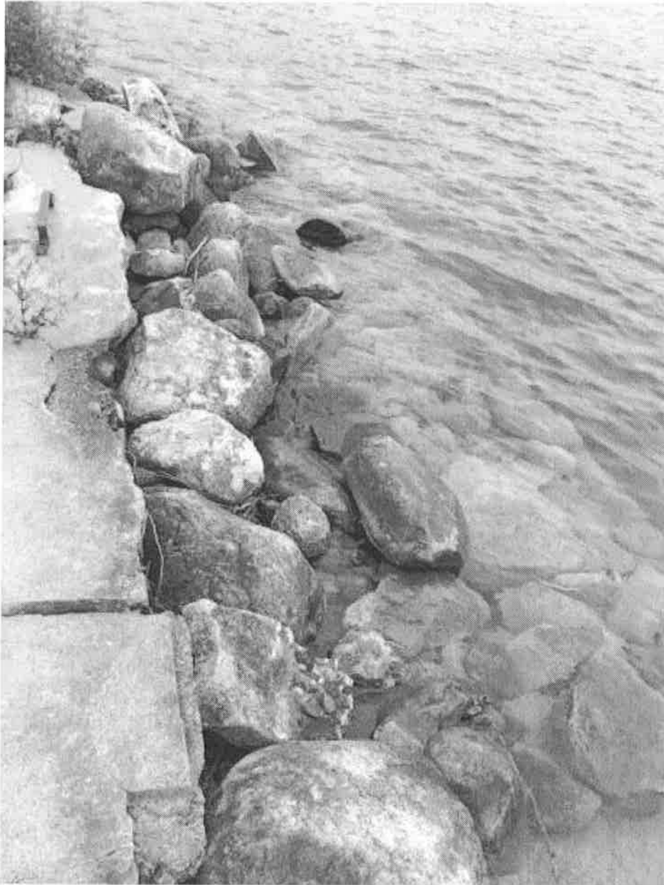
The full length of the crib section of the pier dock, looking—parallel to the shore—from the end of the right side to the end of the left side of the pier dock
