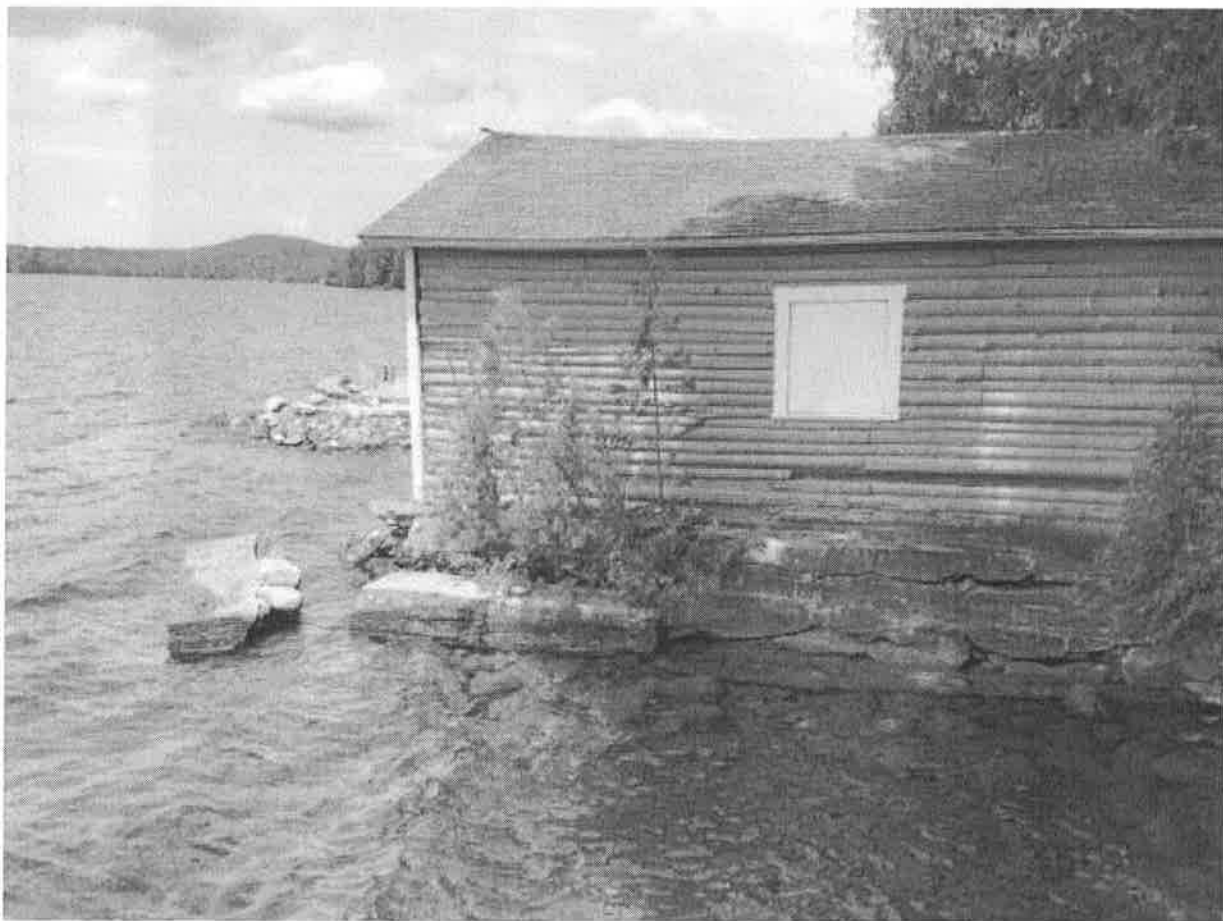
Side view of boathouse, showing detached section of concrete foundation
