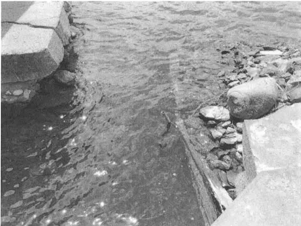
Left side; sagging crib section of the dock blocks passage between dock and boathouse
