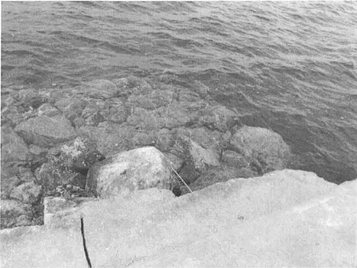
Right front corner, showing where the crib section adjoins the concrete section
