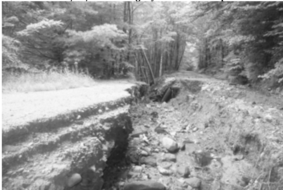
Overlook Road 7/11/2024 This gully was over 8' deep at the far end!
