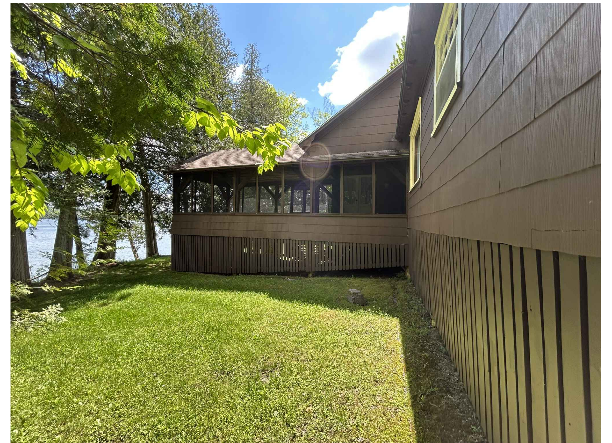
PHOTO OF NORTH SIDE OF EXISTING SCREEN PORCH & NORTHEAST LAWN AREA (LOOKING SOUTH)
