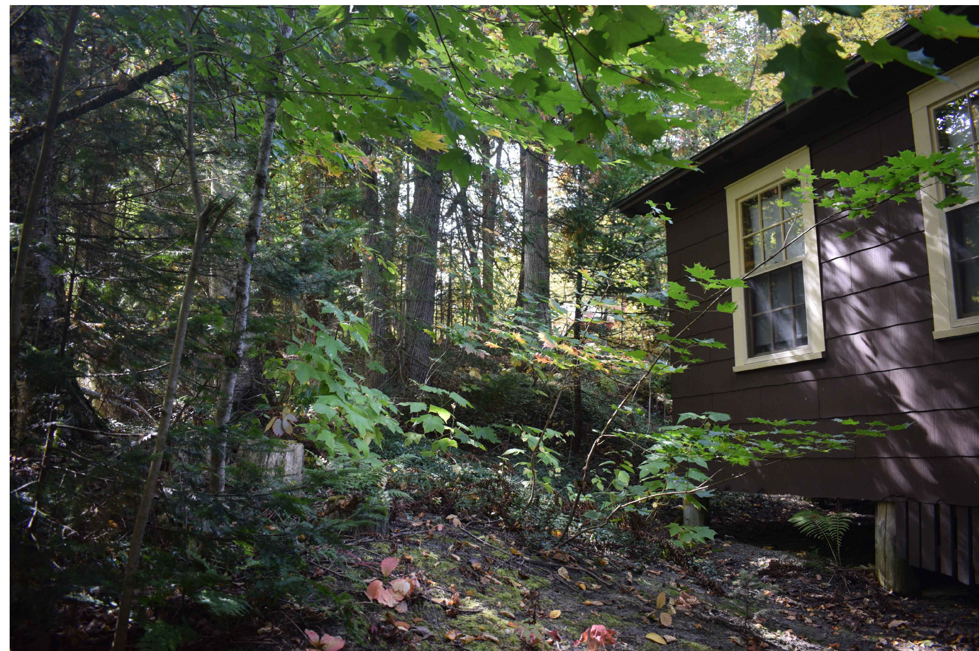
PHOTO OF EXISTING SOUTHWEST HOUSE CORNER LOOKING UPHILL TOWARDS BARRE BOULEVARD & EXISTING SITE VEGETATION (LOOKING WEST)
